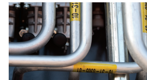
Steel pipework for better heat dissipation
